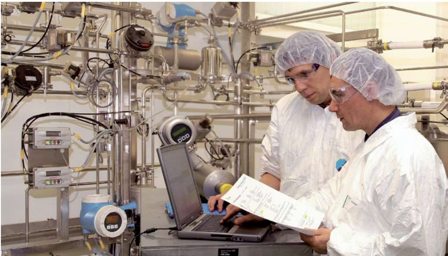
Inventory of critical devices in a pharmaceutical plant
